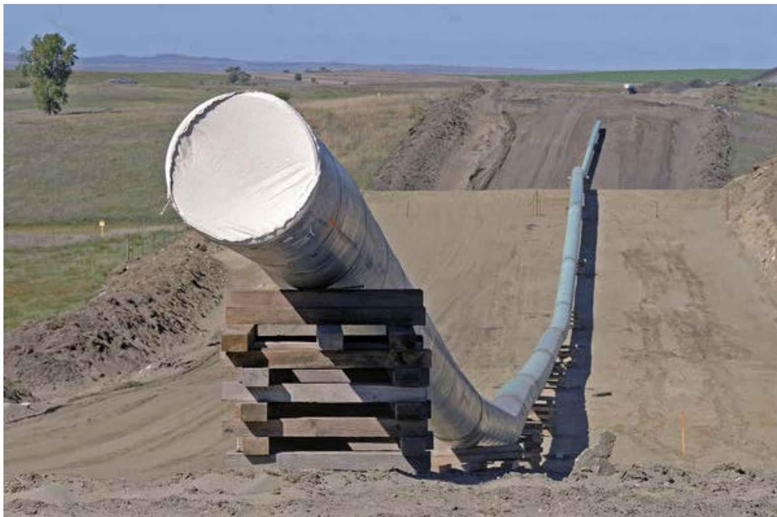
A short section of the Dakota Access pipeline in September 2016. (Tom Stromme / Associated Press)
